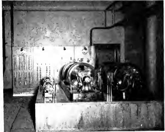
FIG. 2.—POWER PLANT, MAIN EXCHANGE.
